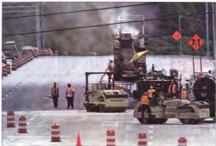
Workers pour part of Interstate 40 in downtown Knoxville in this July 2008 photo. The high price of asphalt means state and local governments are pursuing fewer road projects these days. Bruce Wuesthich, senior director of engineering and public works for Knox County, said the county has not had to sacrifice capital projects — the building of new roads or major reconstruction projects that generally cost more than $50,000. Instead, it has scaled back maintenance projects in subdivisions.
